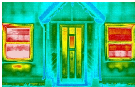
Both windows have radiators on the wall below them. The right-hand window's radiator is fitted with Radflek, which has reduced heat loss through the wall by 45%. This can be seen by the more muted colour below that window compared with below the left-hand window
